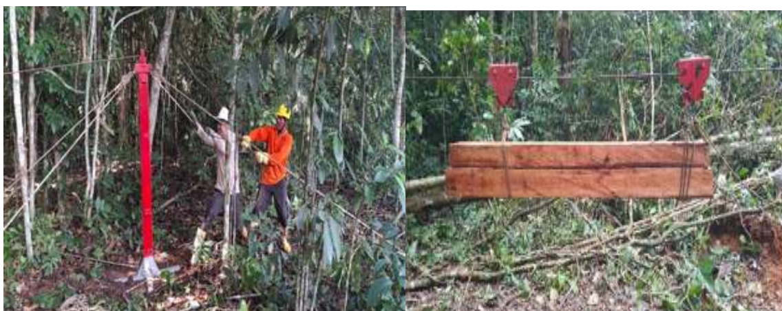
Figure 8. Installation and operation of the medium-height aerial cable at Los Puertos, Calamar NDFyB
